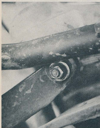
One of the problems we ran across was the forward member of the cantilever rubbing against the pipe. There isn't a hole yet, but we figure there will be soon.
