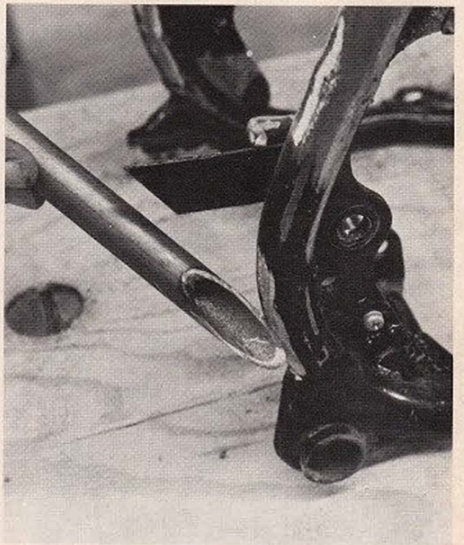
24 With both the new bracing tube and the frame member ground an ideal large welding surface is available. Also clean the bracing ear for welding.
