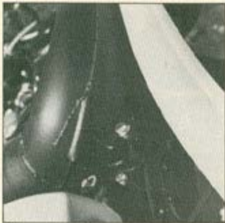
Former trouble spot on the pipe belly has been beefed up to prevent cracking.
