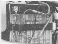
Electrolyte level must be between marks on battery casing
